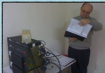
Local pastor, Carlos Puratt, was on hand to help us connect and configure the transmitting equipment. Carlos and his congregation also have TV & Radio stations in their part of town.
